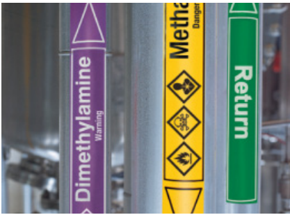
Pipe & valve marking
