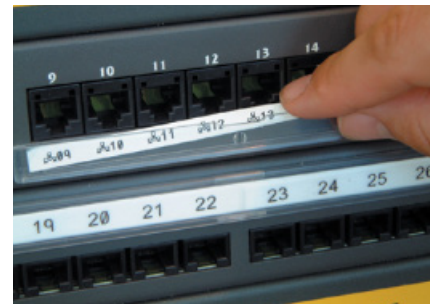
Punch block & patch panel labels
